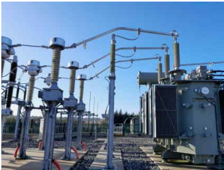
Plate 2-4 Typical 110kV transformer connection
