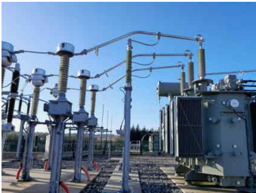
Plate 2-4 Typical 110kV transformer connection
