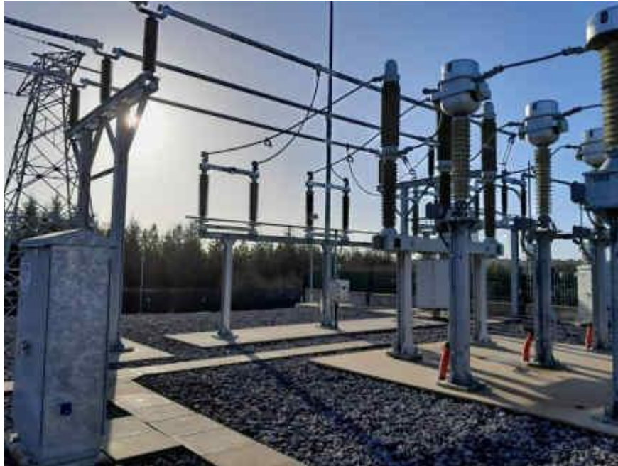
Plate 2-3 Typical 110kV electrical infrastructure
