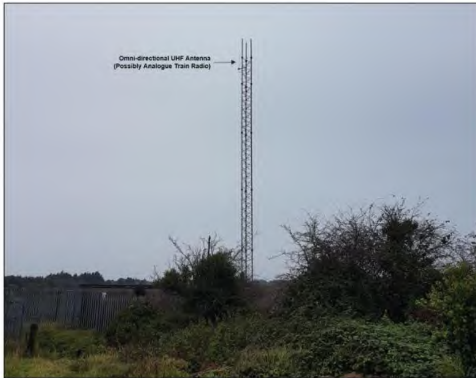
Plate 15-1 Telecoms Mast at Claremorris Train Station
